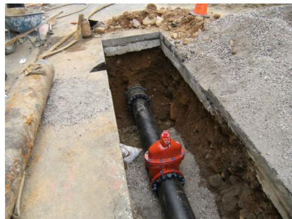
NEW WATER MAIN ON ROGERS AVE BETWEEN EMPIRE BOULEVARD AND STERLING STREET
