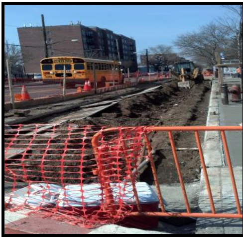
Excavation for bus pad on Nostrand Avenue between Avenue U and Avenue T
