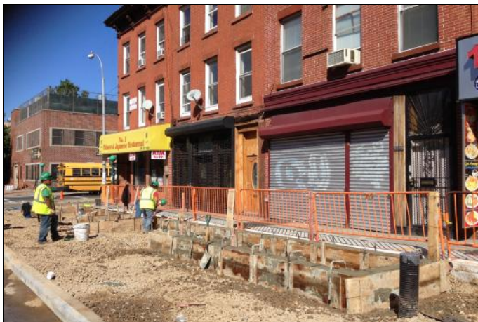
Select Bus Service Bus Stop Construction on Bedford Avenue between Clifton Place and Lafayette Avenue
