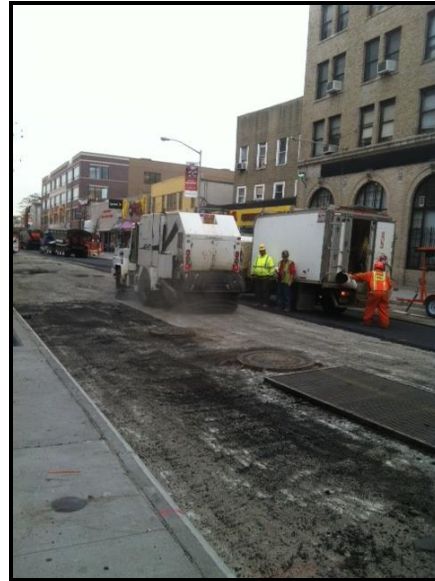
Milling of Roadway - south side Church Avenue between Flatbush Avenue and Bedford Avenue looking east towards Bedford Avenue.
