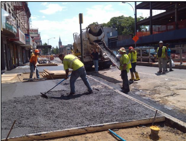
Installation of pigmented concrete sidewalk on Church Avenue between Flatbush Avenue and Bedford Avenue.
