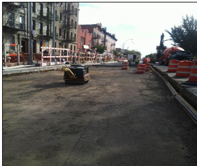
Reconstruction of Roadway on Church Avenue between Bedford Avenue and Rogers Avenue looking East towards Rogers Avenue
