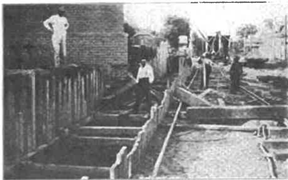
Brighton Beach Line—Method of Excavating for Trench Showing Temporary Supports for Brick Building and Derrick for Handling Earth.
