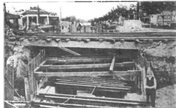
Brighton Beach Line—Trench Excavation for Foster Avenue Sewer Showing Track Supporting Beams before Placing.
