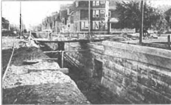
Brighton Beach Line—Retaining Wall, Showing Manhole Opening and Seat for Street-Crossing Bridge.
